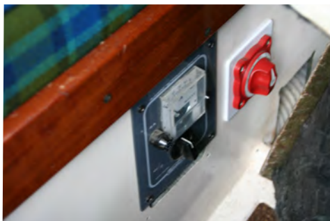
Main Electrical Switch
